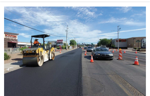
Asphalt paving on 7th Avenue between Thomas Road and Indian School Road.
