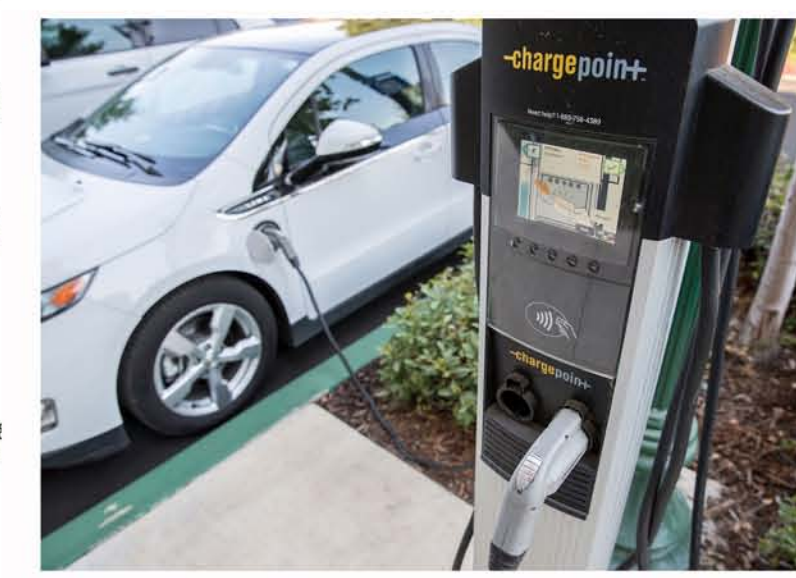
ELECTRIC VEHICLE CHARGING STATION
