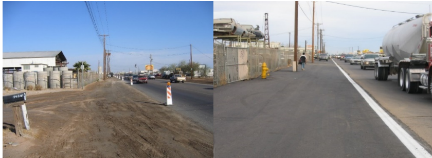
Before and after of surface stabilization on the shoulders of Broadway Avenue.
